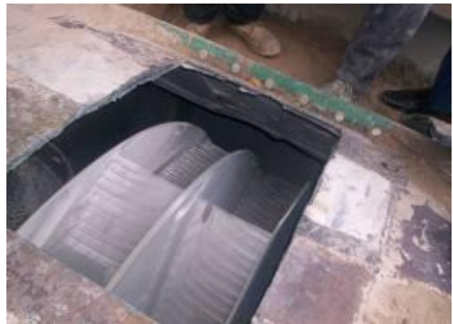
Fan awaiting for repaired
